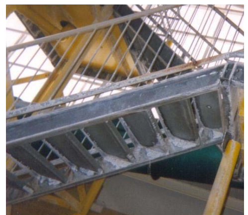
White rusting of heavy duty galvanised steel and red rusting where thin galvanised steel had been used in a new swimming pool complex. Extensive rectification work delayed the opening of the pool and blew out project costs.
