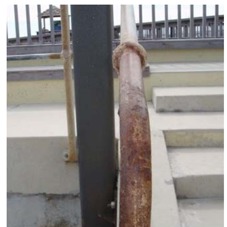
HDG steelwork near a beach was erected less than six years ago. Some sections were coated with an MIO product, which has inhibited corrosion.
