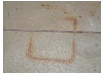
Rust stains on concrete
