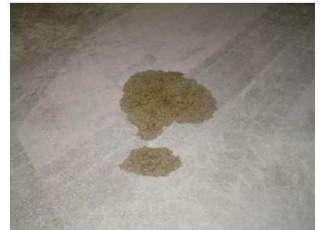
Oil stain and laitance on concrete
