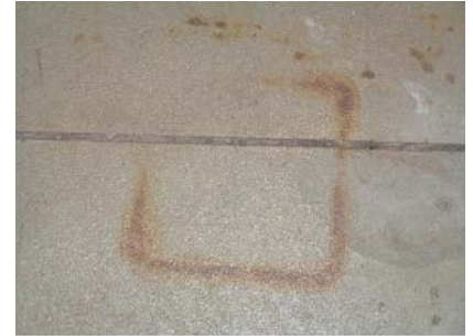
Rust stains on concrete
