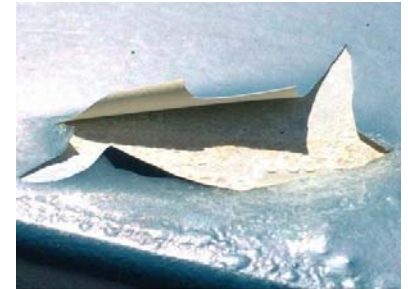
White rusting of zinc layer caused delamination of the coating
