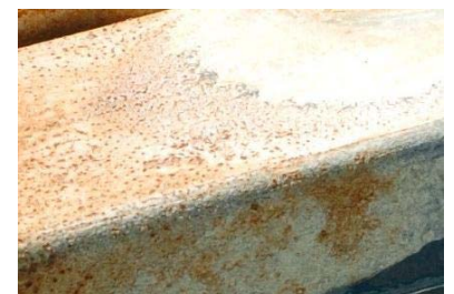
Inadequate zinc layer was quickly depleted, allowing steel substrate to corrode
