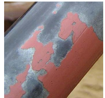
Little or no surface profile on the substrate caused coating failure.
