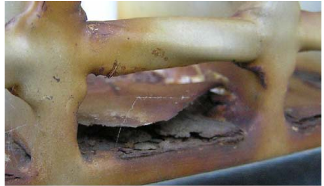
The photo clearly shows the blue-grey millscale causing red rusting of the steel below it and delamination of the heavy-duty coating above. The steel was painted only four years before!
